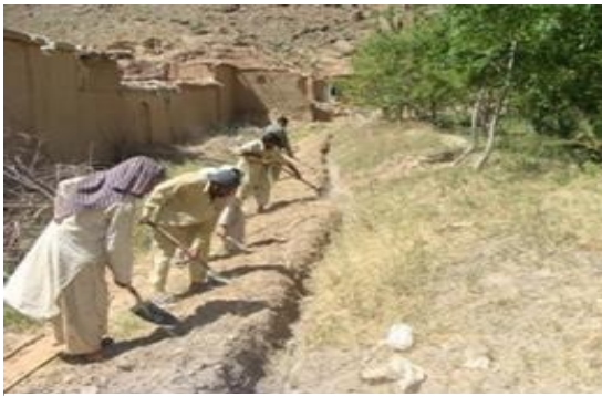
Figure 14: Local labour, under the supervision of skilled field engineers carry out construction and rehabilitation of all infrastructure projects.
